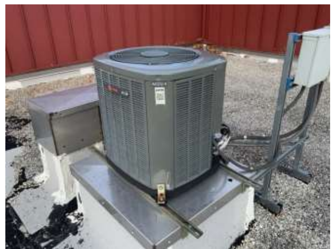
18 - SPLIT SYSTEM HEAT PUMP
