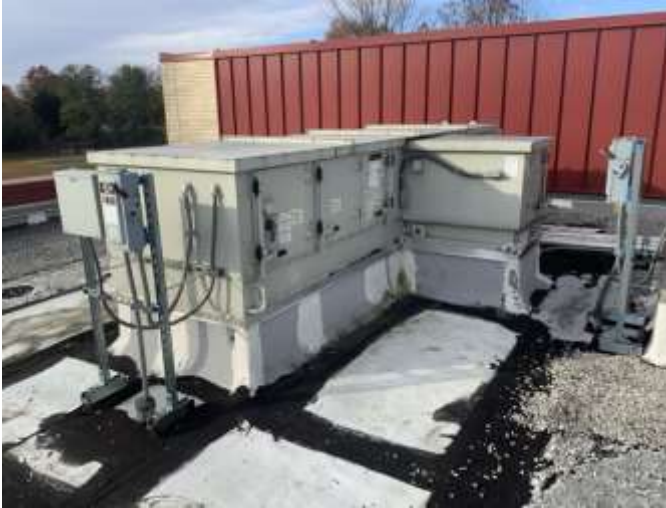
19 - TYPICAL AIR HANDLER
