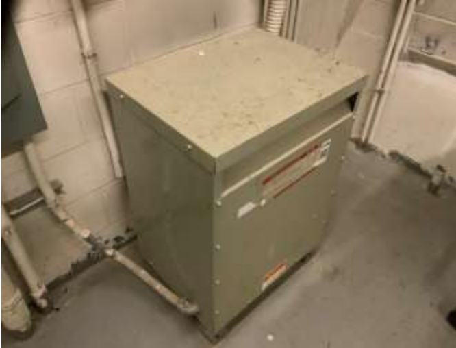
25 - STEP DOWN SECONDARY TRANSFORMER
