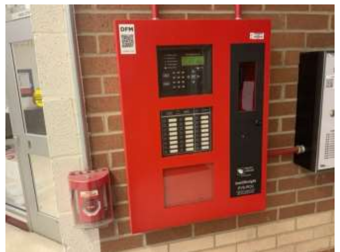
30 - FIRE ALARM PANEL
