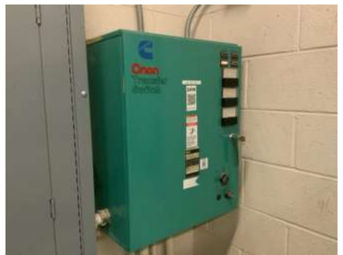
24 - AUTOMATIC TRANSFER SWITCH
