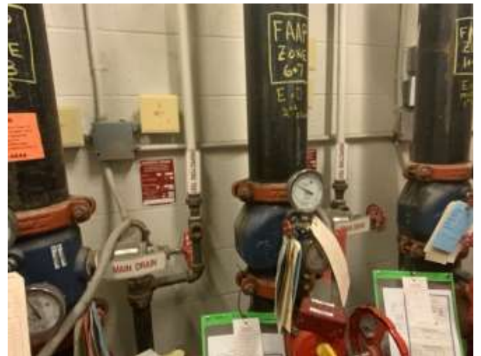
22 - SPRINKLER SYSTEM RISERS
