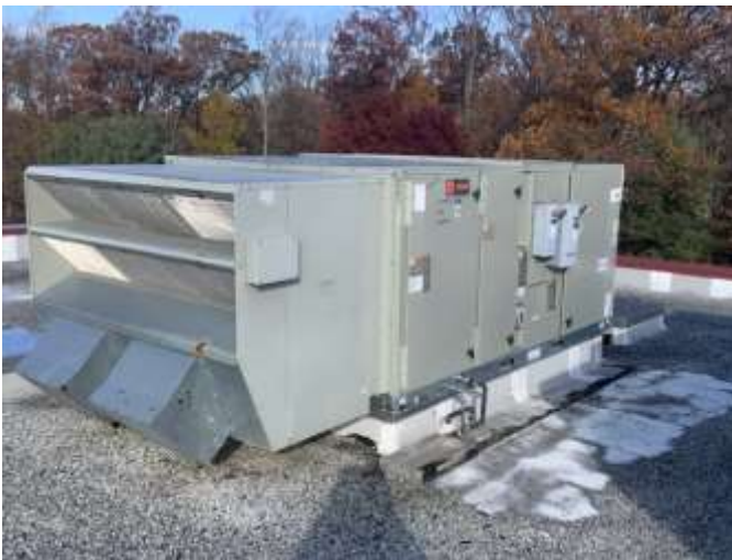
21 - ROOFTOP PACKAGED UNIT
