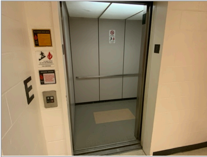
LOBBY LOOKING AT CAB
